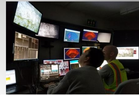
Data Control Room
